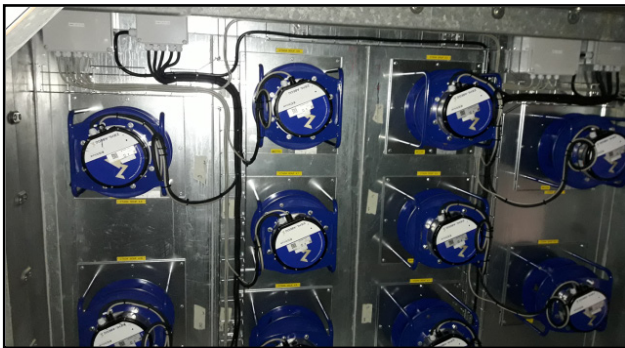
Figure 11. Example of direct drive multi grid fans with EC motors installed
