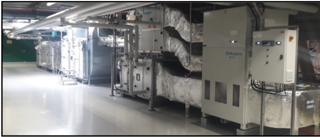
Figure 1. Overview of a typical HVAC of the case study
